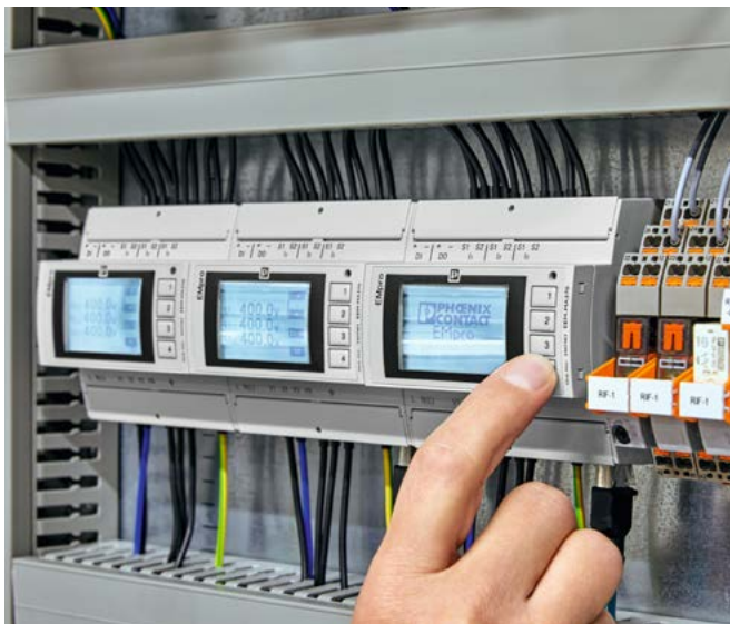
Energy monitoring in the control cabinet is rapidly becoming commonplace.
