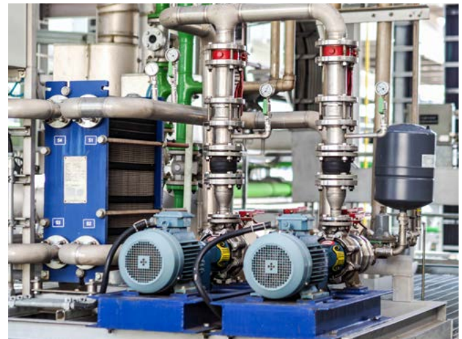
Preventing downtime, saving energy, and improving asset performance are just a few of the benefits of proactively monitoring energy.
